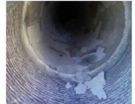
Examples for scaling in hydrogeothermal plants
